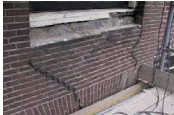
Subsidence as a result of drought
